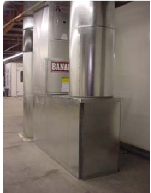
Air Utilities View
