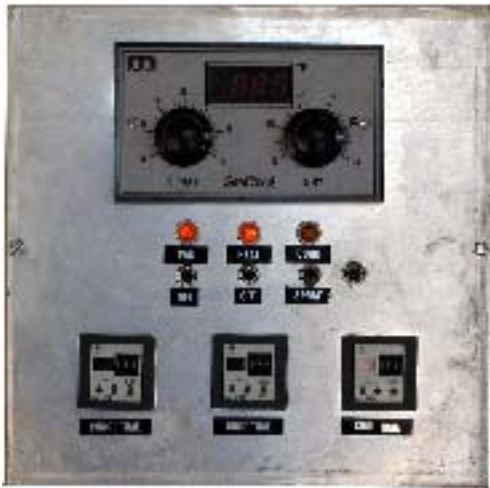
SPRAY CURE CONTROL PANEL
